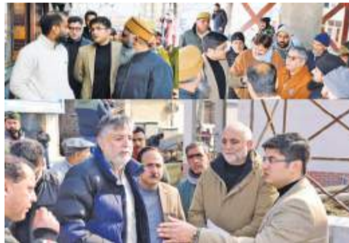
6 THE COMMISSIONER LATER INSPECTED ONGOING WORKS AT THE JHELM RIVERFRONT, with particular focus on the underground cabling project. Terming the Riverfront a high-value urban and tourism asset, he instructed executing agencies to immediately augment manpower and resources to ensure timely completion of works."
