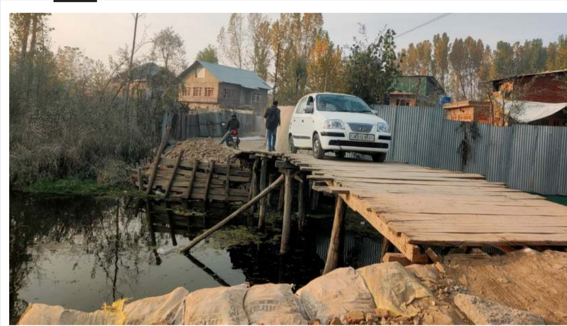
DECAYING PATHWAY: A deteriorating wooden bridge in Mir Behri, Dal, poses a significant risk to commuters and pedestrians. KO PHOTO, SYED MOHAMMAD BURHAN
