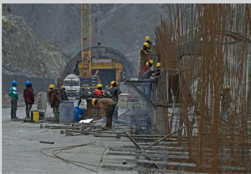
WORKERS RAISE A RETENTION wall at the site of under-construction Zojila tunnel in Sonamarg area of Central Kashmir's Ganderbal district.
