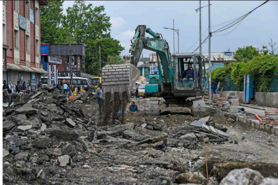
Work under Srinagar Smart City Project on at trendy Residency Road in Srinagar, KO Photo Abid Bhat
