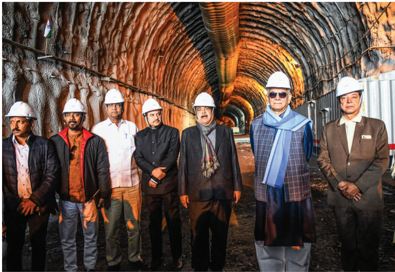
Union Minister of Road Transport and Highways, Nitin Gadkari and J&K Lieutenant Governor, Manoj Sinha pose for a photograph after inspecting the ongoing work on the ambitious Zojila Tunnel project on Monday. KO Photo, Abid Bhat
