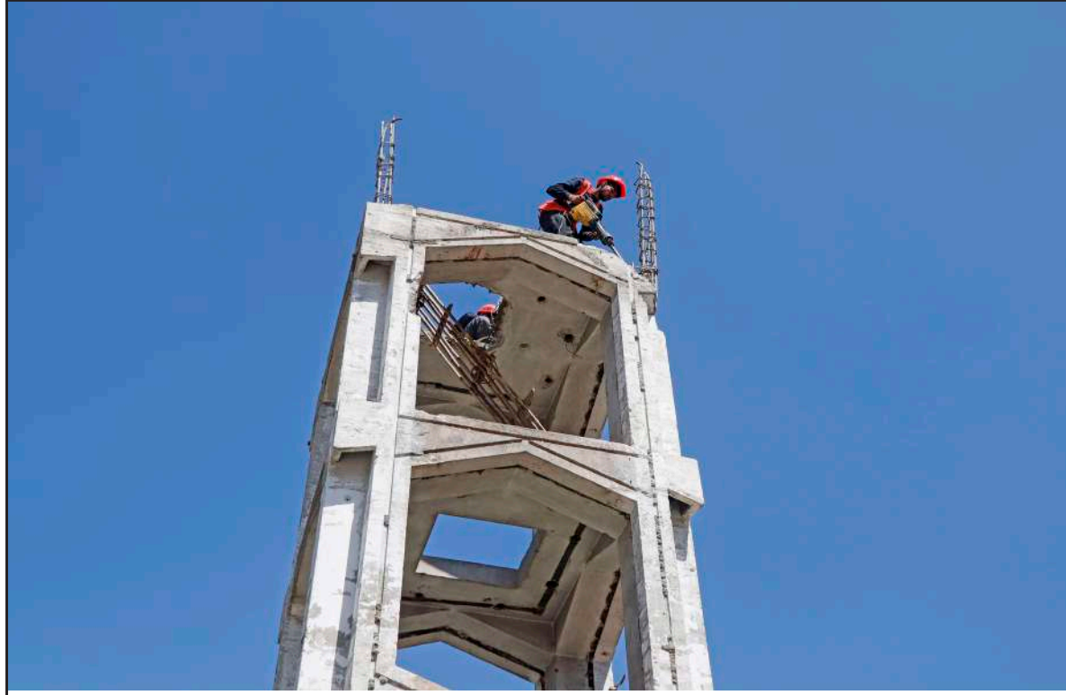
Historic Ghanta Ghar (Clock Tower) undergoes major facelift under Srinagar Smart City Project, KO Photo Abid Bhat
