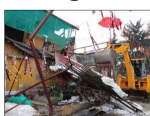
go for any sort of illegal constructions/ encroachments, without obtaining proper building permission from the competent authority. It was given out that strict action in terms of conducting demolitions followed by lodging of FIR's shall be taken against violators who try to raise the constructions in the In-Lake / Green Belt areas.
