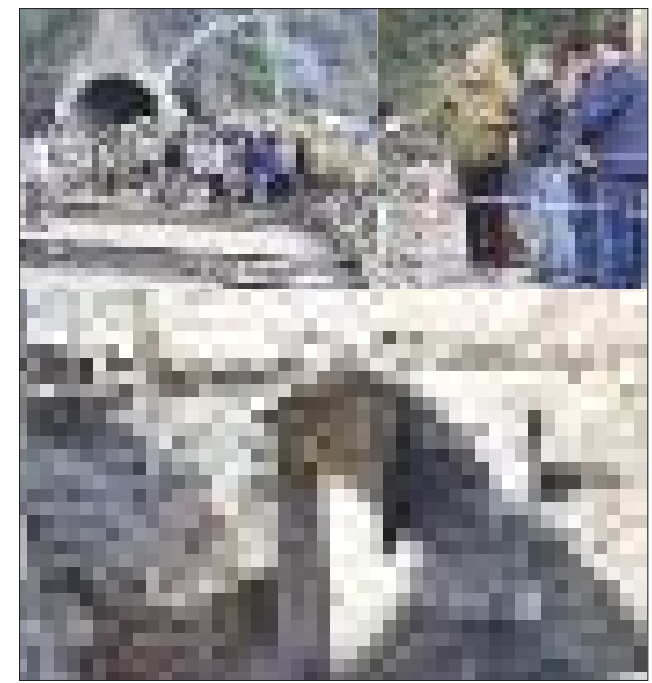
DC Ramban, Nazim Zai Khan inspecting progress on the construction of Bailey Bridge at Kela Morh, Ramban on Thursday. Photo: Info dept
